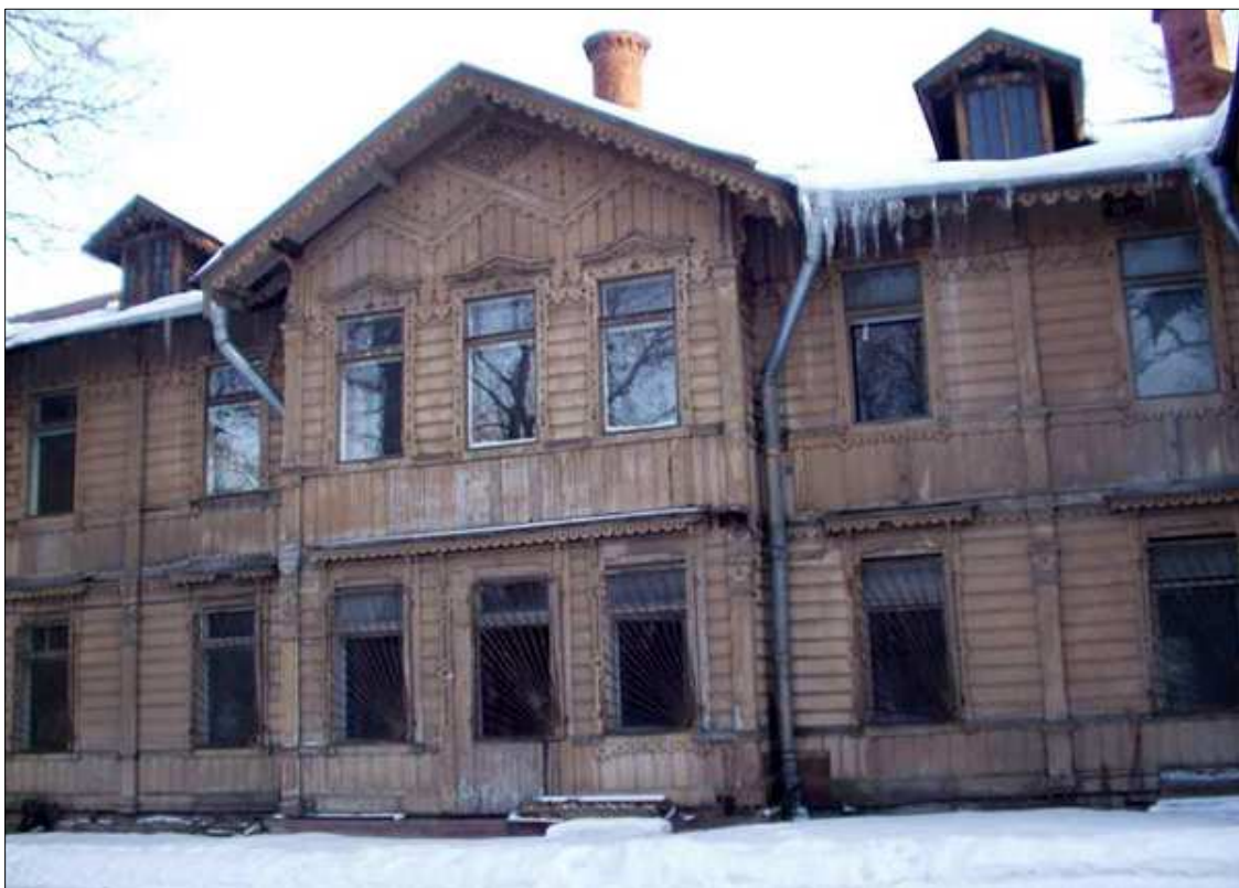
The building of the St. Petersburg city hospital for the mentally ill in the name of Great Martyr and Healer Panteleimon, the current state.
